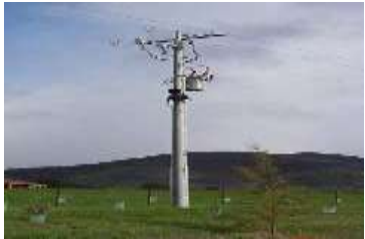
Power Distribution Poles
