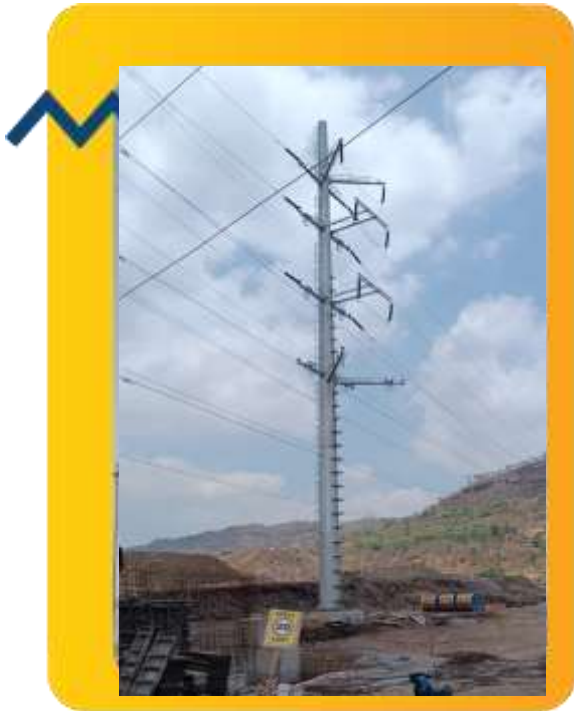
220 kV D/C Poles – Special Pole
