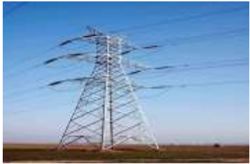
Power Transmission Tower
