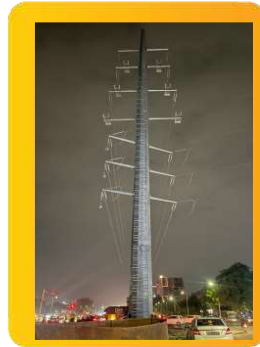
220 kV CT MC Pole - Torrent
