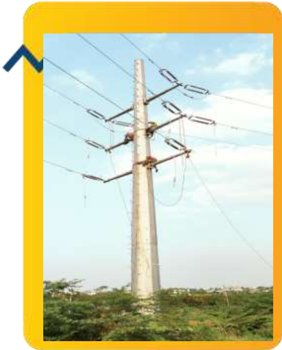
110 kV Embedded Pole
