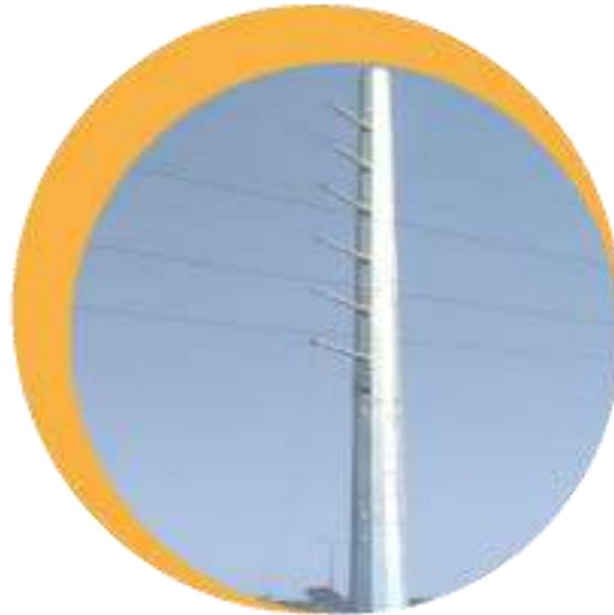
132 kV single sided cross-arm
